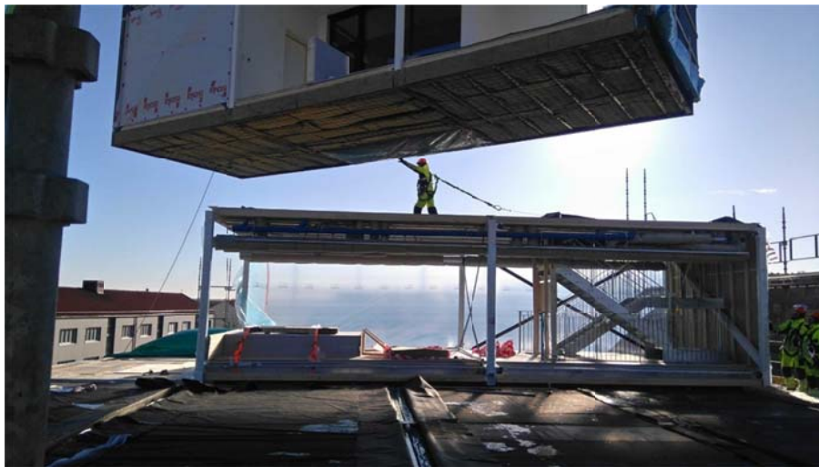
Figure 1: Assembly of HSB Living Lab; placement of 44 modules constructed by Swedish Modules company within 10 days.
