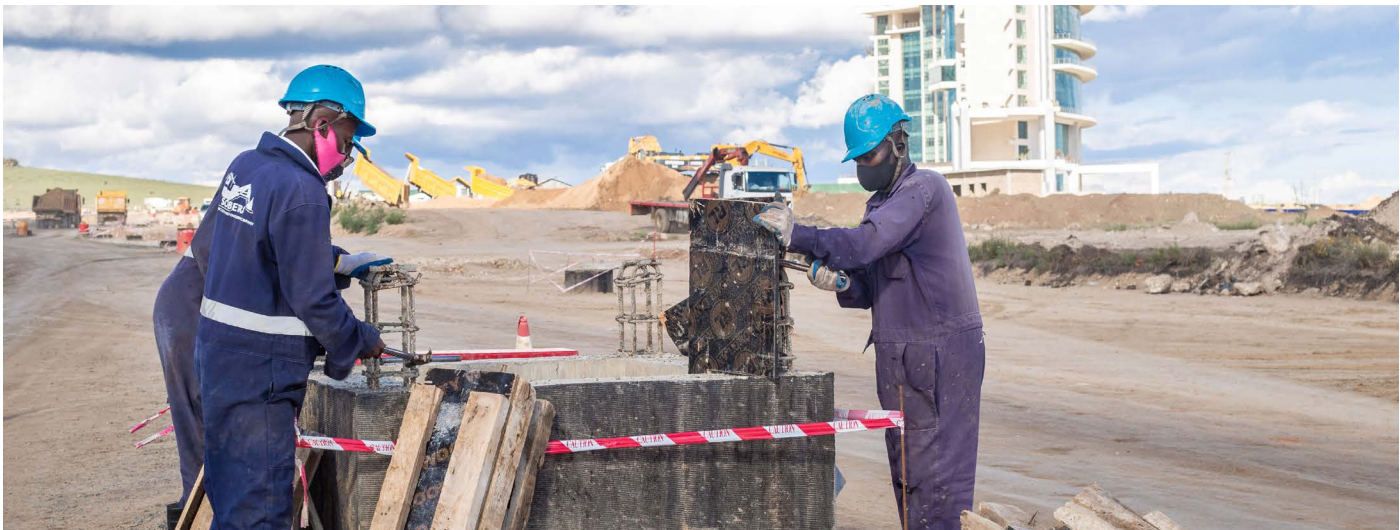
Workers at the ongoing Konza Technopolis. Konza is a key flagship project of Kenya’s Vision 2030 economic development portfolio. Once completed, the hub will be a world-class city, powered by a thriving information, communications and technology (ICT) sector, superior reliable infrastructure and business friendly governance systems.
